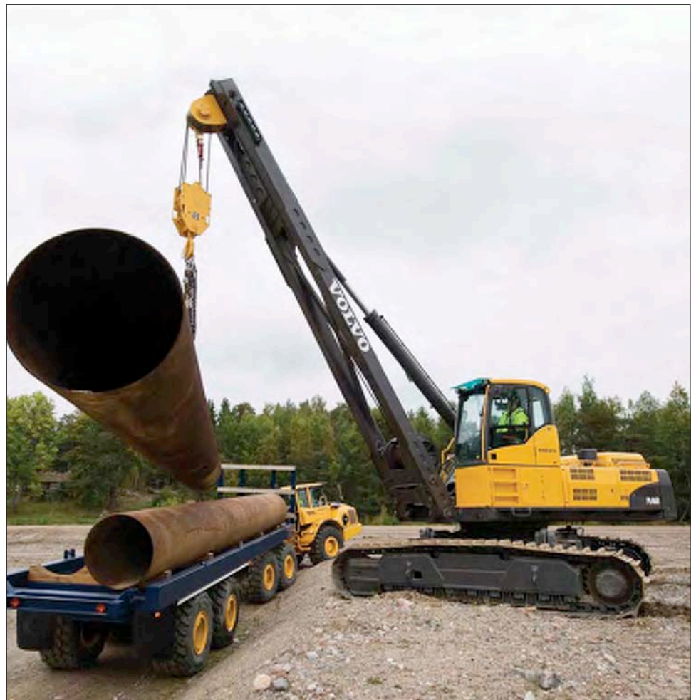
The size of a pipelayer is determined by the size and weight of the pipe being installed and the terrain conditions on the jobsite. Large-scale transmission pipelines will require larger machines, while distribution projects are better suited for smaller and midsize machines.
